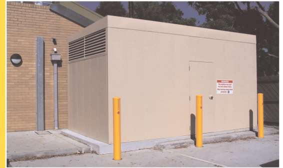
Beneath this sound-proofed outer lies another noise attenuating enclosure to ensure the Olympian generator does not disturb the peace.
